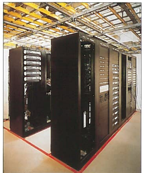
The new amplifier racks.
